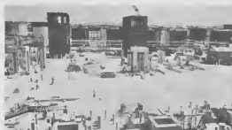
Work progressing on Hydrogen unit in April 1970. View from Powerhouse No. 1 looking north.
